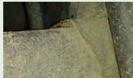
Crack in suspension.
