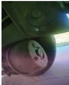
Suspension hanger cracked. Photo by Brad Billington.
