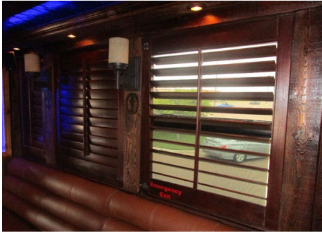
Exit obstructed by wooden plantation shutters.
